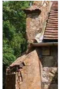
Detail of a crumbling corner buttress to which stonework repairs were made
